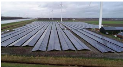
11.75MW Netherlands, 2019 Centrale photovoltaïque bifaciale de type N
